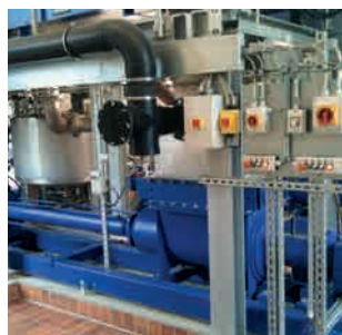
Conveyance of sludge from decanter to silo: KL65RÜ80.4 Progressive cavity pump with fill level monitoring
