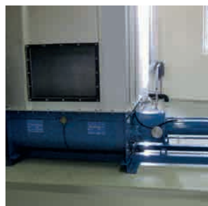
Conveyance of dewatered sewage sludge from decanter for drying: KL65R80.2 Triplex progressive cavity pump
