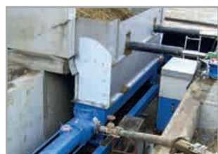
WANGEN KL-R pumps in operation
