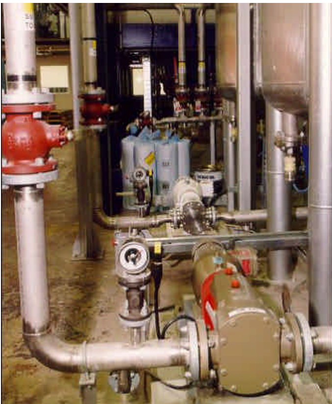
Series D4 pump handling UV resin with Series S3 pump handling water-base ink in background at printing ink plant in UK
